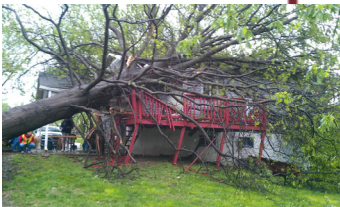
Damage from Tornado, 2011.
